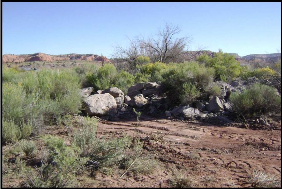
Parcel 12 / AOC 93 – Bivouac and Tank Training Area – South debris pile area removal up to rocks to remain in place
